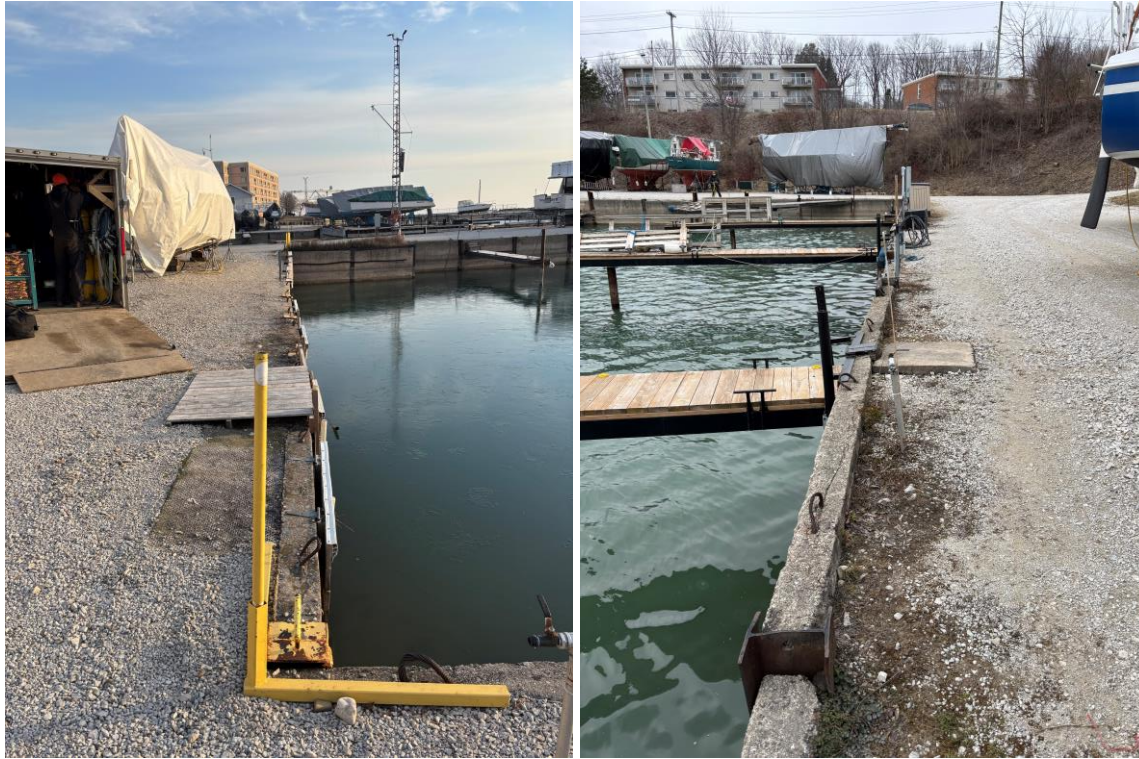
Photo 3.16 Leaning of Basin Walls at S4 (Left) and S13 (Right) (10/04/2025)
