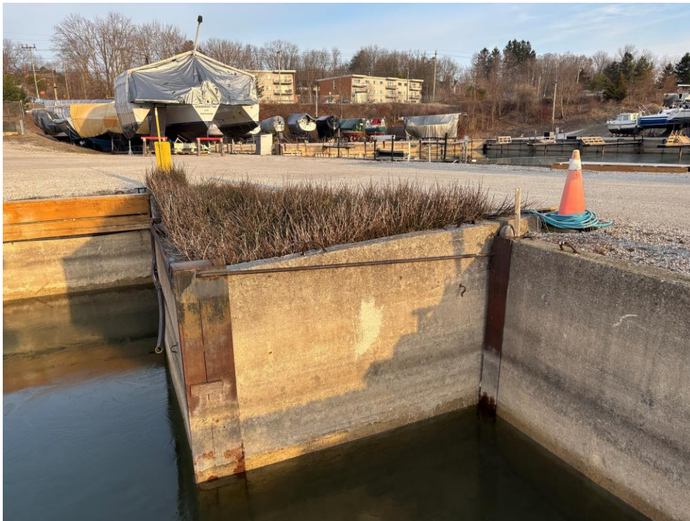
Photo 3.15 Tilted Concrete Panel (10/04/2025)
