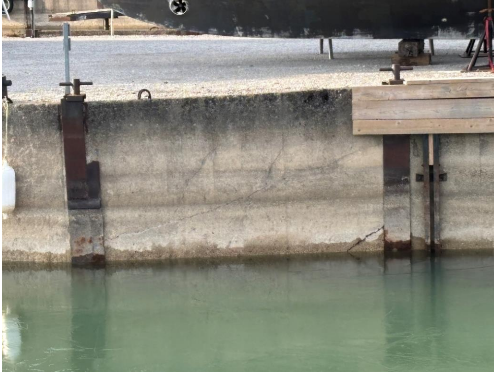
Photo 3.14 Cracking and Tilting of Concrete Panel (10/04/2025)
