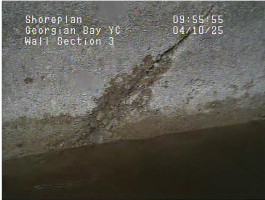
Photo 3.24 Cracking of Concrete Panel (10/04/2025)
