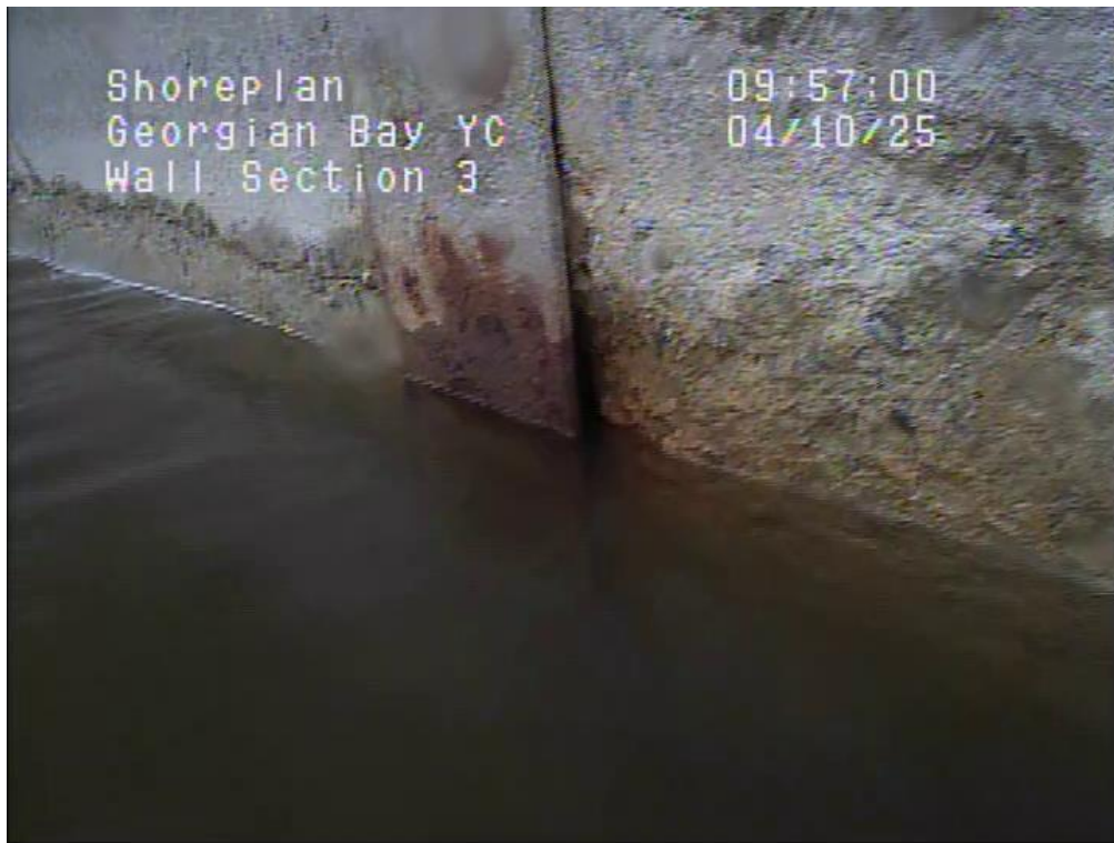
Photo 3.23 Cracking of Concrete Panel (10/04/2025)
