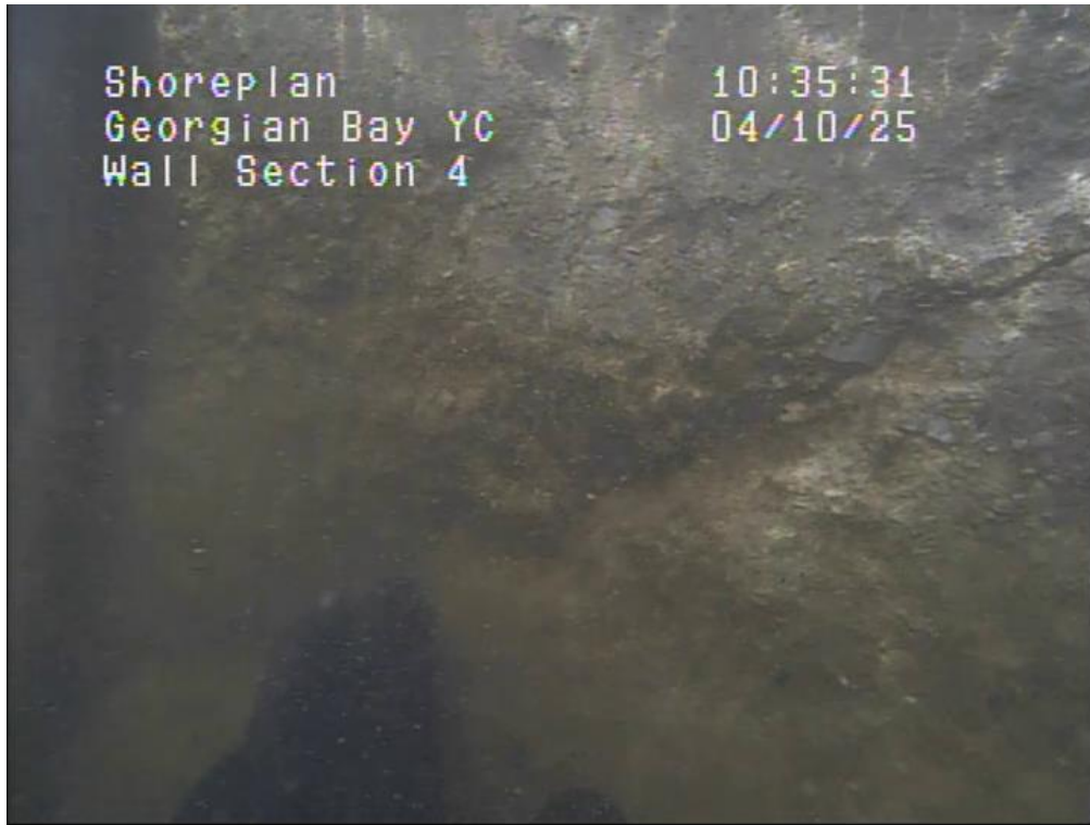
Photo 3.22 Spalling of Concrete Panel (10/04/2025)
