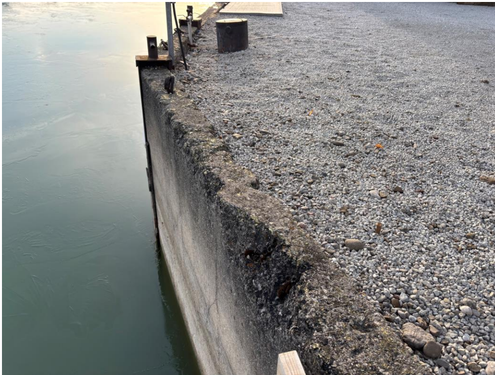
Photo 3.13 Spalling of Concrete Panel at S10 (10/04/2025)
