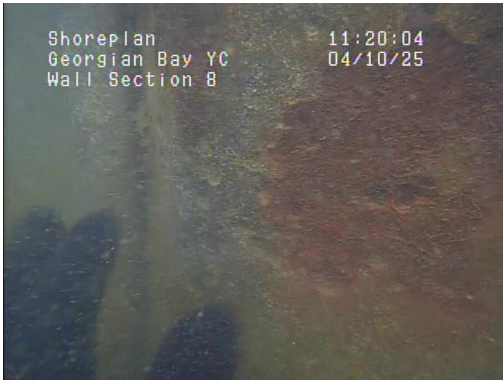
Photo 3.26 Rusting and Pitting of SSP (10/04/2025)
