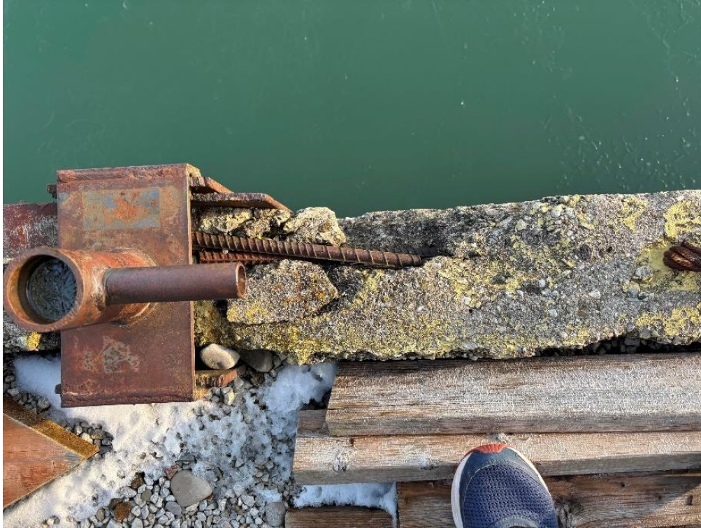
Photo 3.12 Exposed Concrete Panel Rebar at S9 (10/04/2025)
