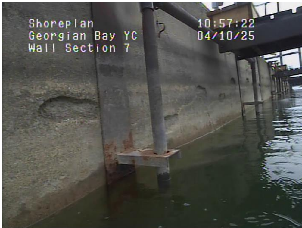
Photo 3.25 Footprints in Concrete Panel at S7 (10/04/2025)
