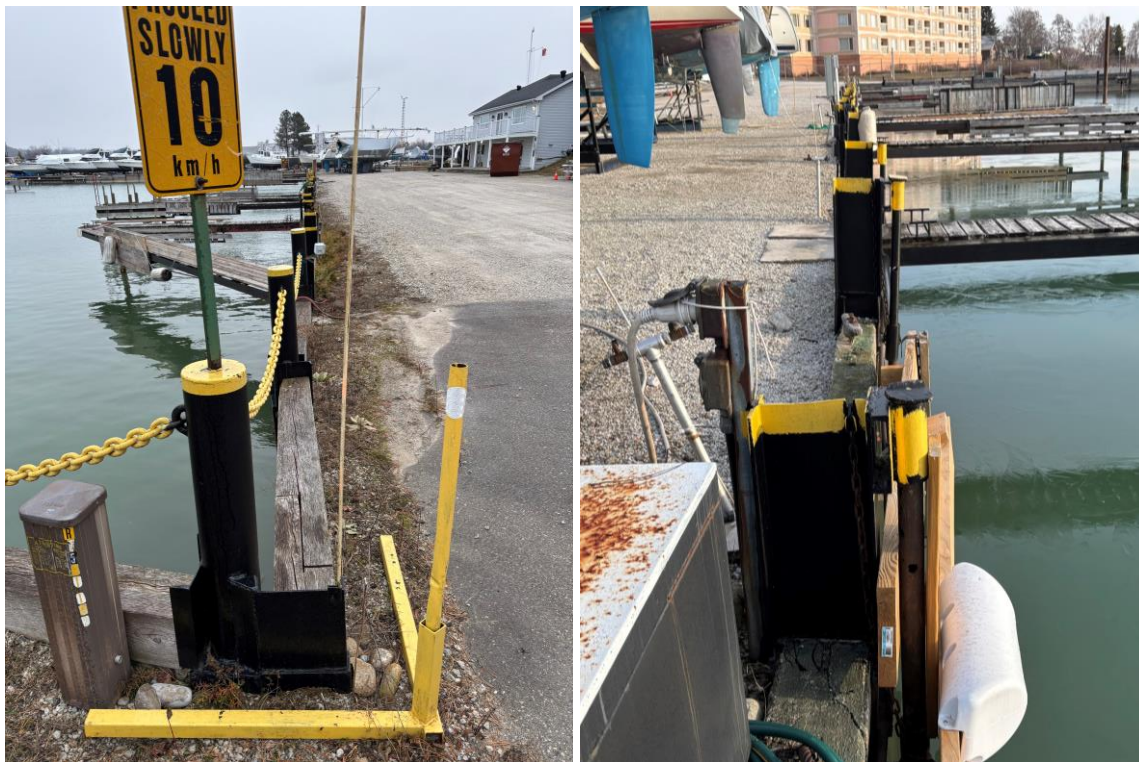
Photo 3.17 Leaning of North Basin Wall at S16 (10/04/2025)
