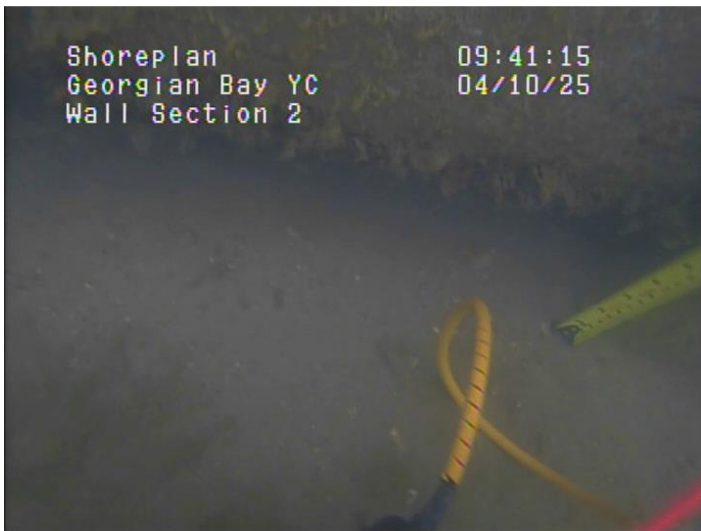
Photo 3.21 Gap Between Concrete Panel and Lake Bottom (10/04/2025)
