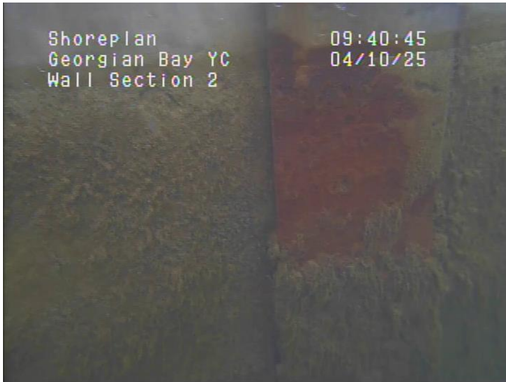
Photo 3.20 Typical Rusting of KP at Water Line (10/04/2025)
